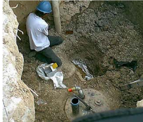
↑Technician Repairs Fiberglass UST at Central Freight lines Facility in San Antonio, TX.
