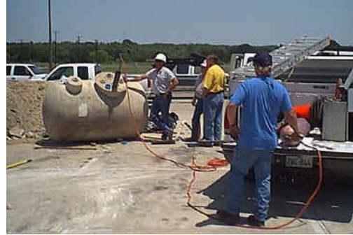
↑Technicians Pressure Test Fiberglass UST After Repairs Complete at Judson I.S.D. Facility in Converse, TX.
