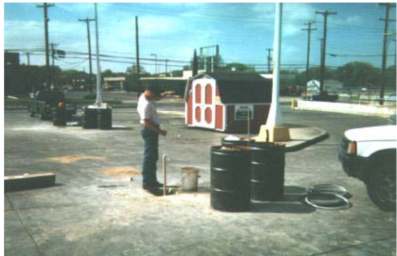
Technician Develops Monitoring Well at Sears and Roebuck Store in Corpus Christi, TX.
